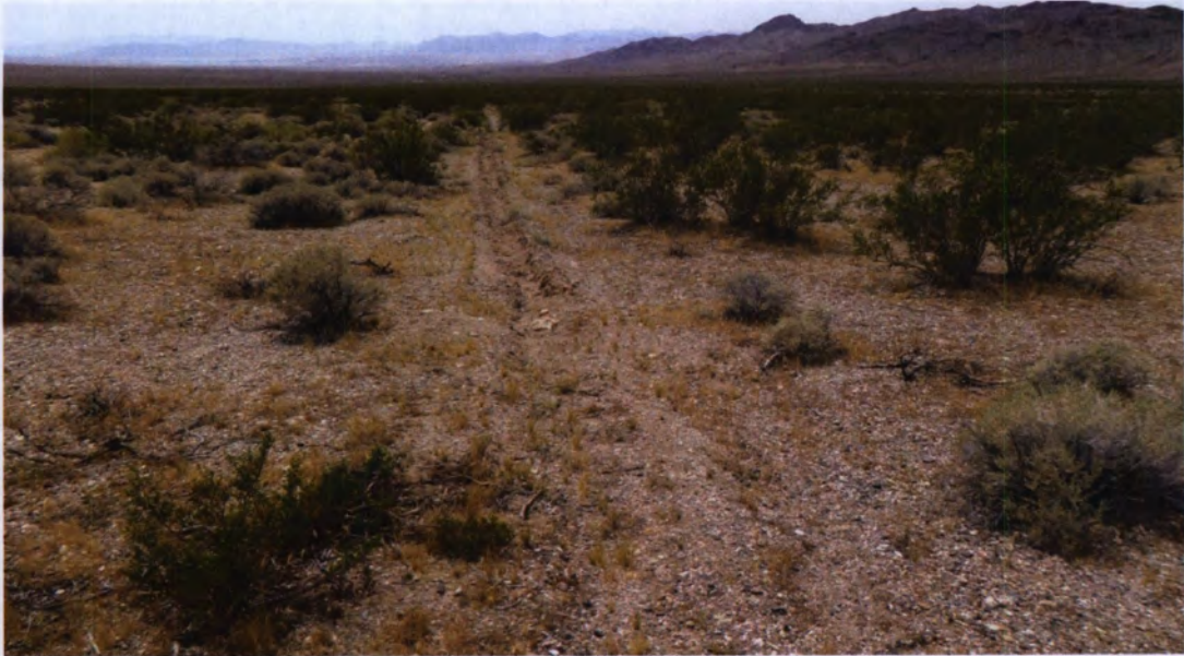
Image 14: Trench and pipe #3 continue southwest toward Fisherman Cove area. Photo looking southwest. Photographed May 10, 2015.
