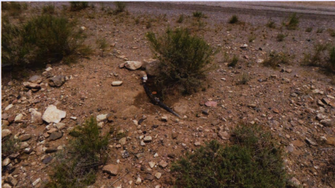
Image 13: Pipe #3 and valves just west of Gold Butte road. Must have used an existing pipe to cross under the road. This pipe and valve have water but the new water trough is still dry. Photo looking east. UTM 11 S 749561 4053233. Photographed May 10, 2015.
