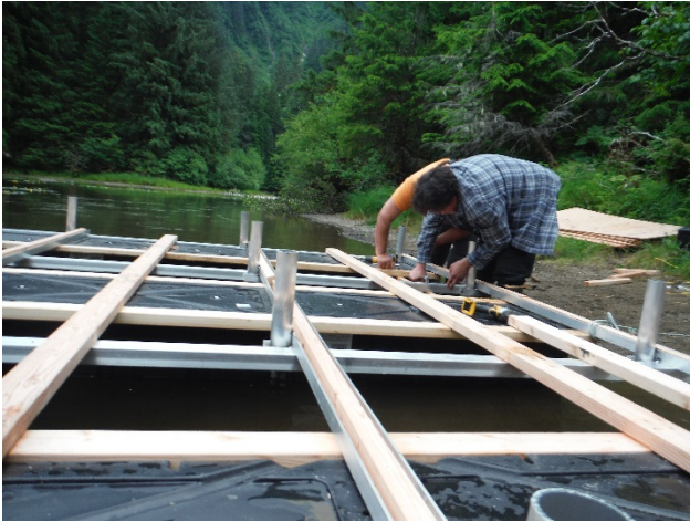
Figure 1. Rebuilding the raft for the floating wall tent at Kook Lake, July 26, 2017.
