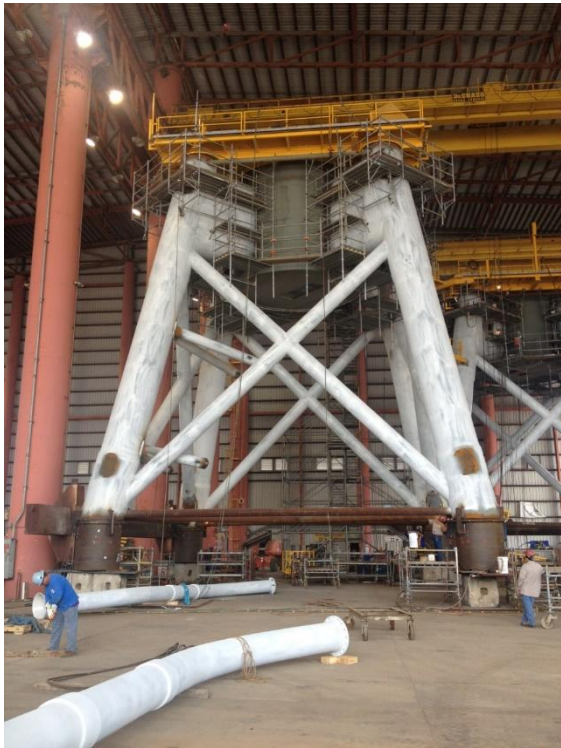
Fabrication of Block Island Foundations by Gulf Island Fabricators, in Houma, LA
