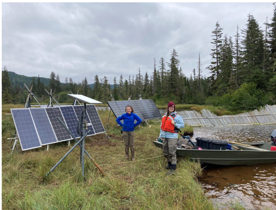
Figure 3. SCA intern Chaney Haavik (left) and USFS fisheries technician Juliet Harrison in front of the newly installed Starlink system at the Sitkoh Lake weir.
