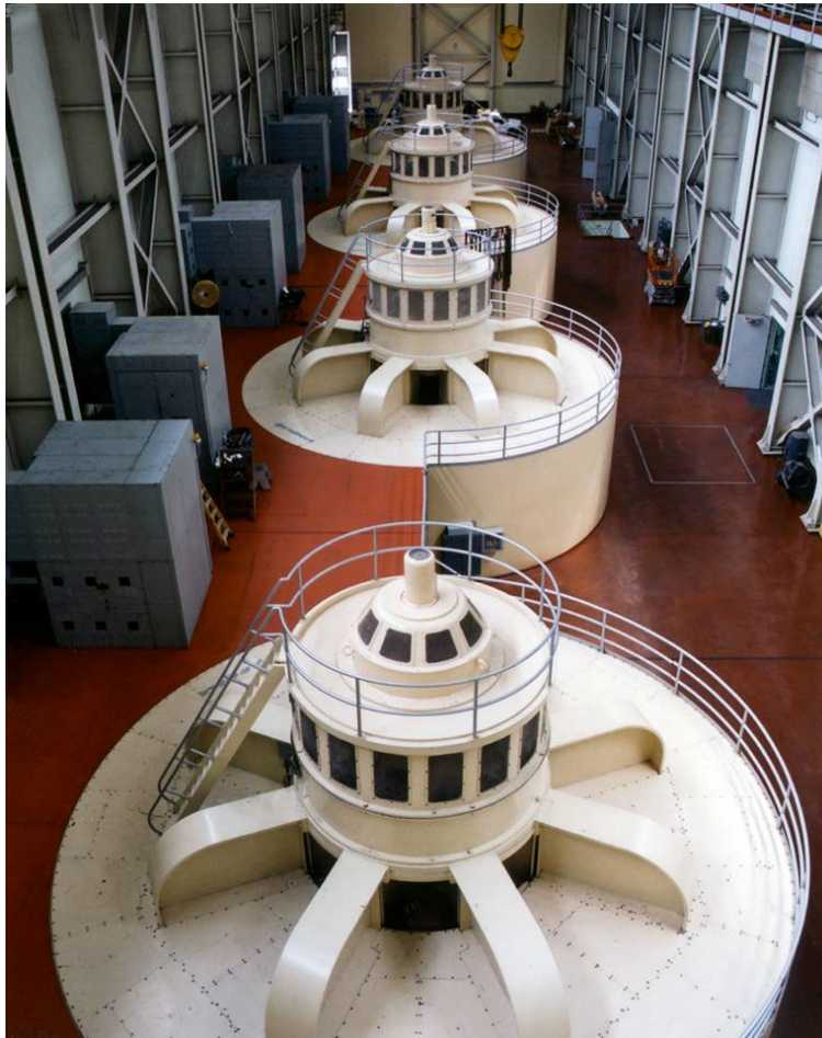
HYDROPOWER TURBINES AT HUNGRY HORSE POWER PLANT NEAR HUNGRY HORSE, MONTANA. RECLAMATION FACILITIES PROVIDE HYDROPOWER FOR MILLIONS OF U.S. HOUSEHOLDS, AND ITS RESEARCH AND DEVELOPMENT WORK FINDS SOLUTIONS TO KEEP BOTH WATER AND POWER FLOWING. PHOTO: BUREAU OF RECLAMATION
