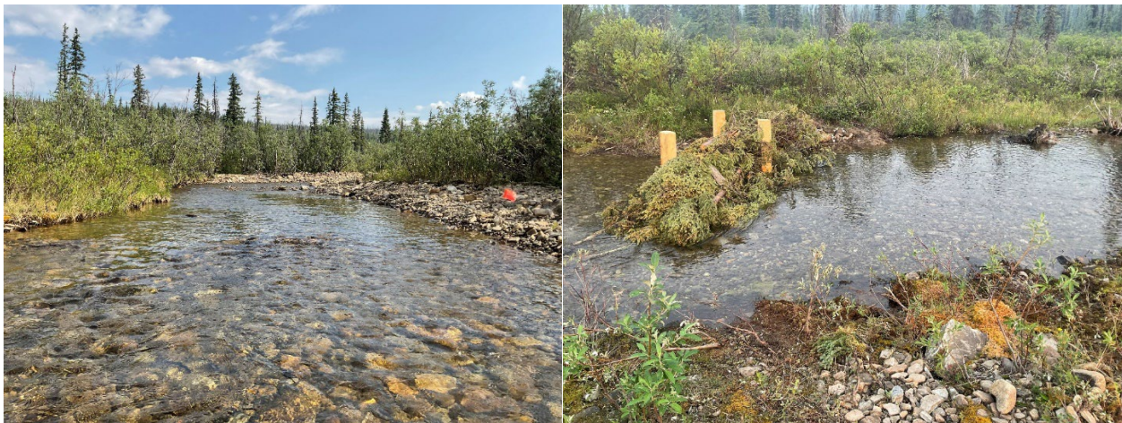
Figure 2. Post assisted structure simulates a fallen tree and is locked in with posts to ensure the material remains in place. This structure produces a point bar downstream and redirects flow to the opposite side, creating a more sinuous stream rather than a straight channel. Over time, the structure will assist in creating diverse pool habitat. This process can take years and the desired outcome is dependent on many environmental factors which control the rate of progress. Left: before & Right: after
