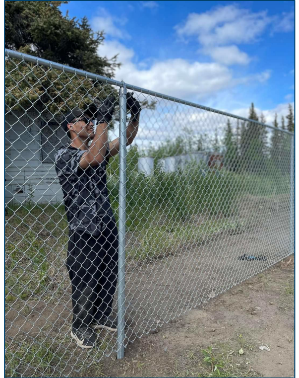
Photo, Trent Adams works on fence in Beaver, Alaska (2022), by Dorothea Adams, CATG.
