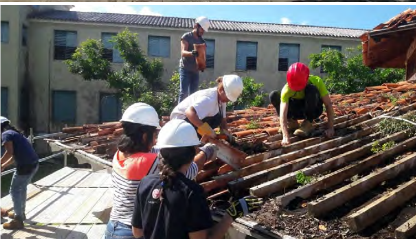
From top: A craftsman repairs an intricate fresco; a restored home in historic Old San Juan; construction workers mend a roof. All images by Héctor J. Berdecía-Hernández courtesy of Escuela Taller.
